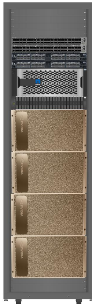
4 DGX A100 systems 1 AFF A800 storage system 1 NS224 disk shelf 2 SN3700V Ethernet switches 2 QM7800 IB switches
